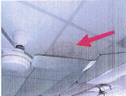
Ceiling Tiles : remove and replace all visibly impacted ceiling tiles throughout remediation areas, ensure source(s) of water intrusion have been repaired by qualified contractor
