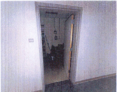
Storage 2 : perform small particle cleaning on exposed surfaces throughout entire area; porous contents with any visible growth should receive small particle cleaning or be discarded
