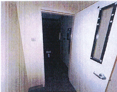
Classroom 8 : perform small particle cleaning on exposed surfaces throughout entire area, steam clean or remove all carpet; porous contents with any visible growth should receive small particle cleaning or be discarded
