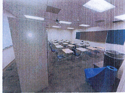
Classroom 10 : perform small particle cleaning on exposed surfaces throughout entire area, steam clean or remove all carpet; porous contents with any visible growth should receive small particle cleaning or be discarded
