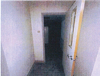
Classroom 10 : perform small particle cleaning on exposed surfaces throughout entire area, steam clean or remove all carpet; porous contents with any visible growth should receive small particle cleaning or be discarded
