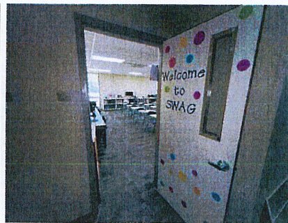
Classroom 6 : perform small particle cleaning on exposed surfaces throughout entire area, steam clean or remove all carpet; porous contents with any visible growth should receive small particle cleaning or be discarded
