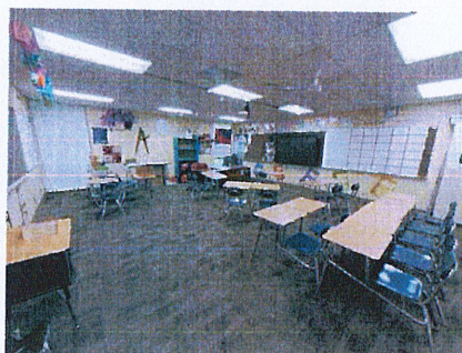
Classroom 14 : perform small particle cleaning on exposed surfaces throughout entire area, steam clean or remove all carpet; porous contents with any visible growth should receive small particle cleaning or be discarded
