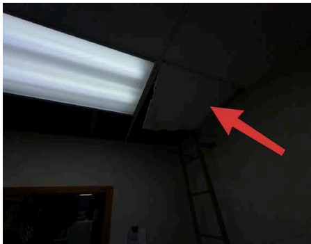
Storage 3 : remove and replace all visibly impacted ceiling tiles throughout remediation areas, ensure source(s) of water intrusion have been repaired by qualified contractor
