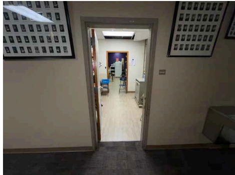
Storage 3 : perform small particle cleaning on exposed surfaces throughout entire area; porous contents with any visible growth should receive small particle cleaning or be discarded
