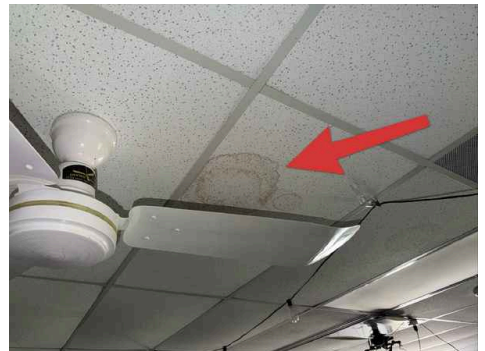
Ceiling Tiles : remove and replace all visibly impacted ceiling tiles throughout remediation areas, ensure source(s) of water intrusion have been repaired by qualified contractor
