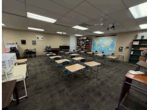
Classroom 7 : perform small particle cleaning on exposed surfaces throughout entire area, steam clean or remove all carpet; porous contents with any visible growth should receive small particle cleaning or be discarded
