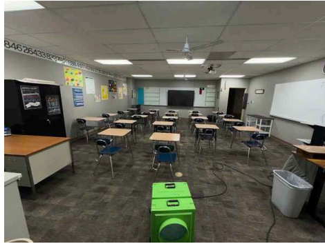
Classroom 8 : perform small particle cleaning on exposed surfaces throughout entire area, steam clean or remove all carpet; porous contents with any visible growth should receive small particle cleaning or be discarded
