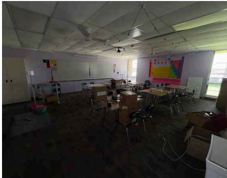
Classroom 17 : perform small particle cleaning on exposed surfaces throughout entire area, steam clean or remove all carpet; porous contents with any visible growth should receive small particle cleaning or be discarded
