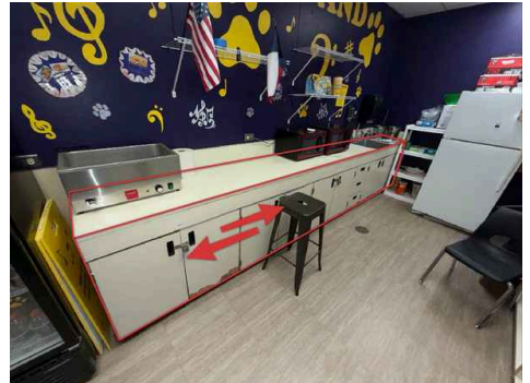
Concession Stand : remove impacted cabinets and drywall behind, clean all exposed framing; perform small particle cleaning on exposed surfaces throughout entire area; porous contents with any visible growth should receive small particle cleaning or be discarded
