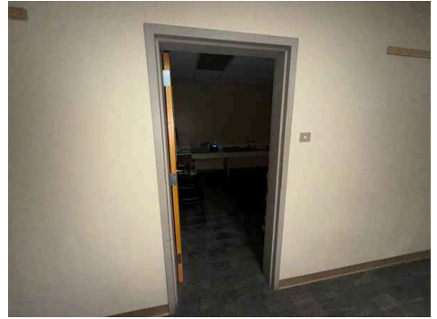
Classroom 9 : perform small particle cleaning on exposed surfaces throughout entire area, steam clean or remove all carpet; porous contents with any visible growth should receive small particle cleaning or be discarded
