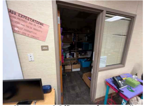
Classroom 6 Office : perform small particle cleaning on exposed surfaces throughout entire area, steam clean or remove all carpet; porous contents with any visible growth should receive small particle cleaning or be discarded
