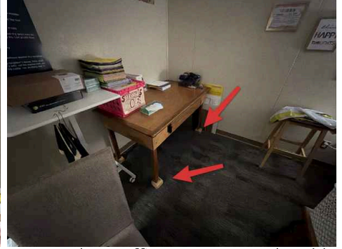
Counselor's Office 2 : suspected mold growth observed
