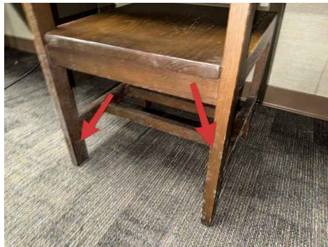
Library : suspected mold growth observed
