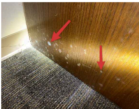
Classroom 7 : suspected mold growth observed
