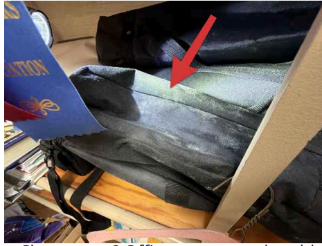
Classroom 6 Office : suspected mold growth observed
