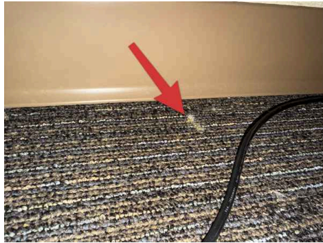
Computer Lab : suspected mold growth observed
