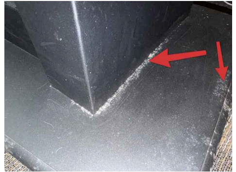
Computer Lab : suspected mold growth observed
