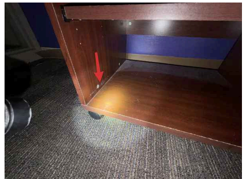
Library : suspected mold growth observed
