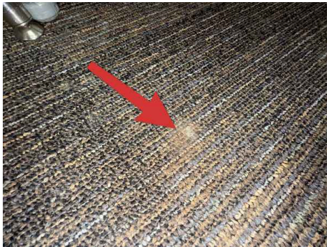
Classroom 2 : suspected mold growth observed
