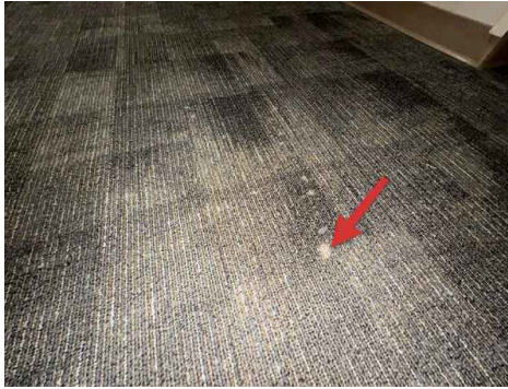
Hallway : suspected mold growth observed
