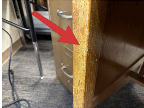
Classroom 3 : suspected mold growth observed
