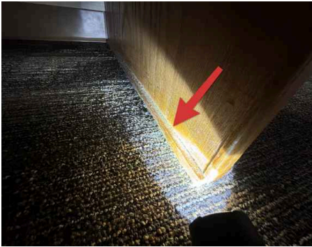
Computer Lab : suspected mold growth observed
