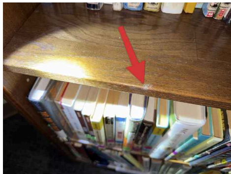
Library : suspected mold growth observed
