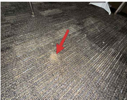
Classroom 2 : suspected mold growth observed
