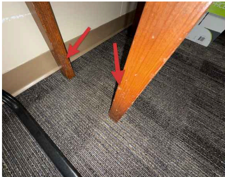
Classroom 9 : suspected mold growth observed
