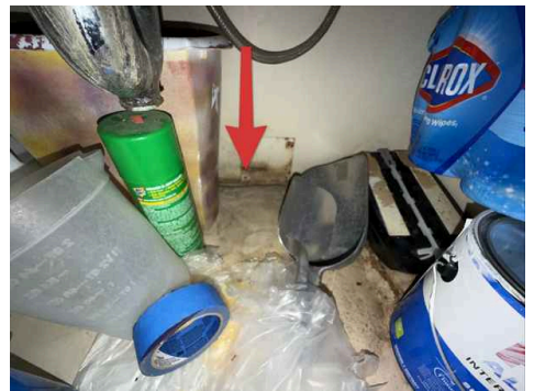
Concession Stand : water impacted material and suspected mold growth observed
