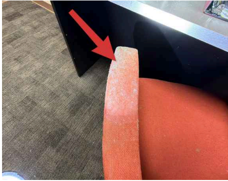
Classroom 6 Office : suspected mold growth observed
