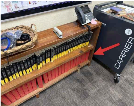
Classroom 3 : suspected mold growth observed
