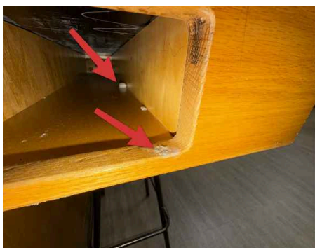
Classroom 16 : suspected mold growth observed
