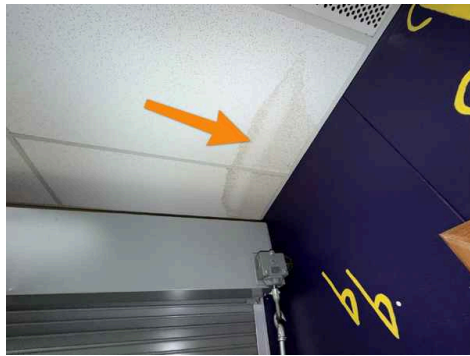
Concession Stand : water impacted material observed
