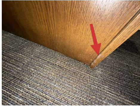
Classroom 13 : suspected mold growth observed
