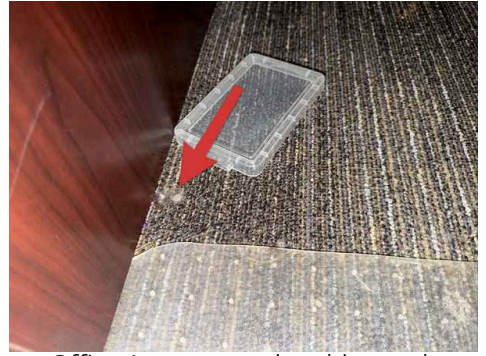
Office A : suspected mold growth observed
