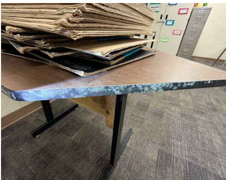
Classroom 1 : suspected mold growth observed
