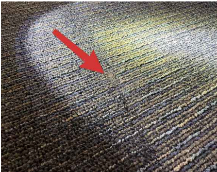
Classroom 2 : suspected mold growth observed
