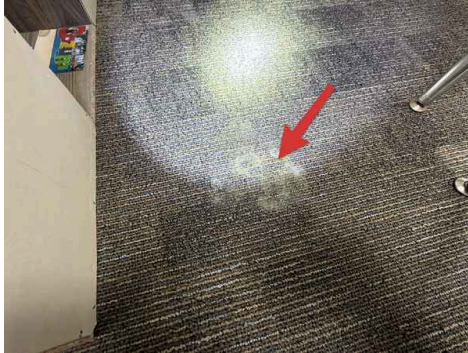
Classroom 2 : suspected mold growth observed
