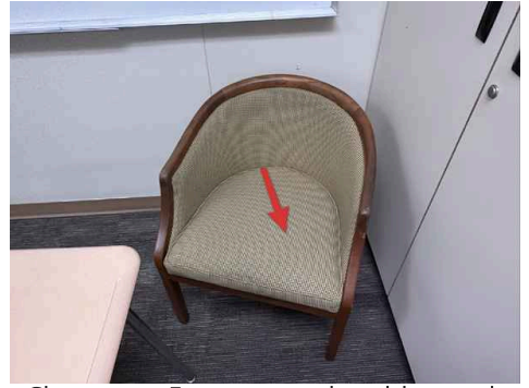
Classroom 5 : suspected mold growth observed
