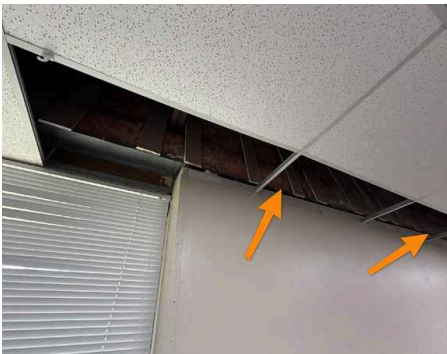
Classroom 5 : water impacted material observed
