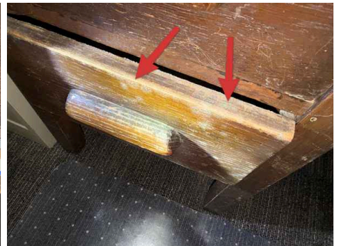
Classroom 7 : suspected mold growth observed
