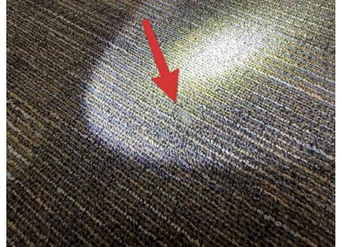
Classroom 2 : suspected mold growth observed
