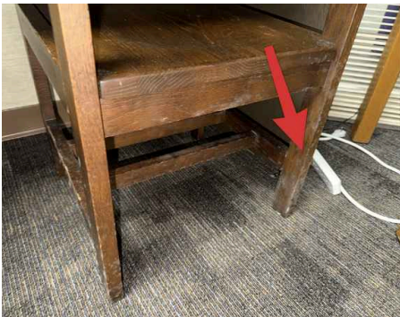
Library : suspected mold growth observed
