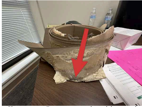
Classroom 5 : suspected mold growth observed
