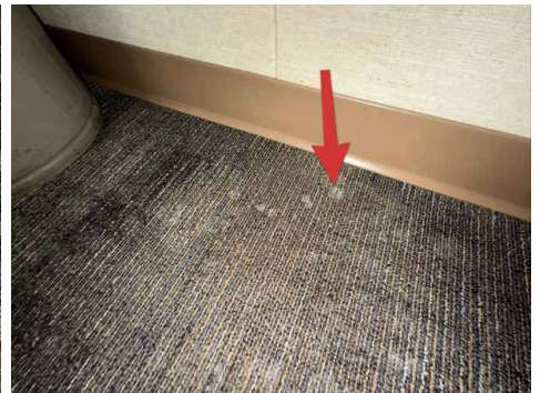
Classroom 14 : suspected mold growth observed
