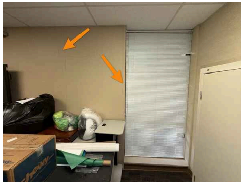
Classroom 15 : water impacted material observed
