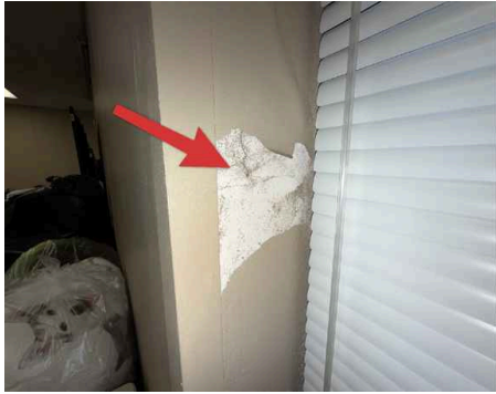
Classroom 15 : water impacted material and suspected mold growth observed
