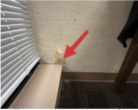
Classroom 1 : water impacted material observed
