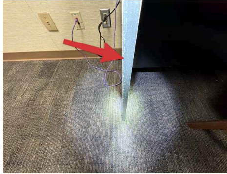
Classroom 6 Office : suspected mold growth observed
