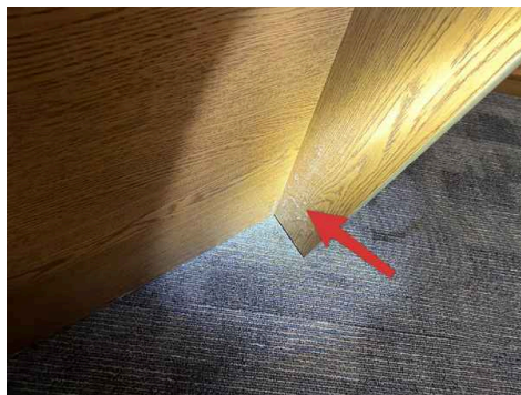
Classroom 1 : suspected mold growth observed
