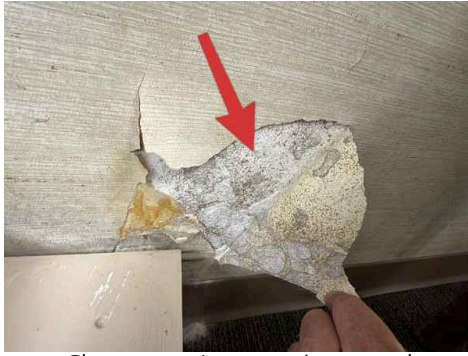
Classroom 1 : water impacted material and suspected mold growth observed
