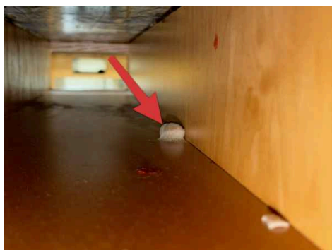
Classroom 16 : suspected mold growth observed
