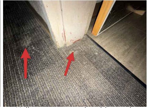
Hallway : suspected mold growth observed
