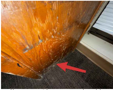
Classroom 12 : suspected mold growth observed
