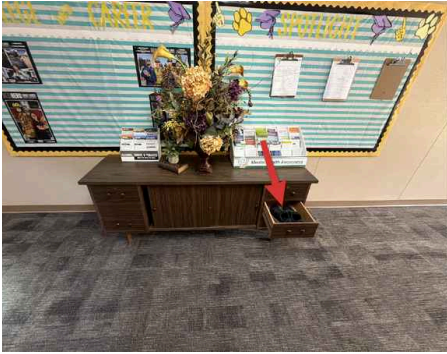
Hallway : suspected mold growth observed
