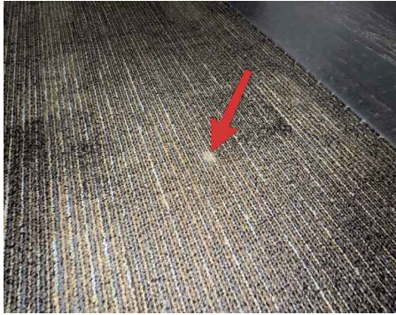
Classroom 13 : suspected mold growth observed
