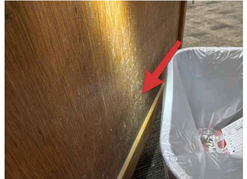
Classroom 3 : suspected mold growth observed
