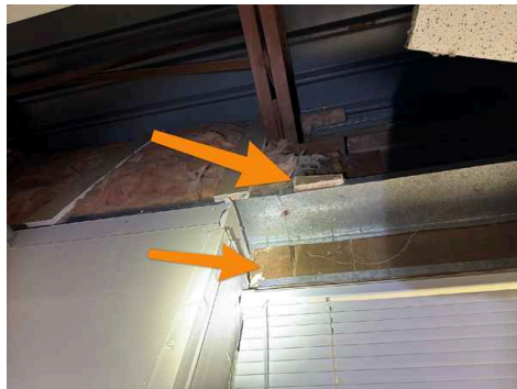
Classroom 5 : water impacted material observed
