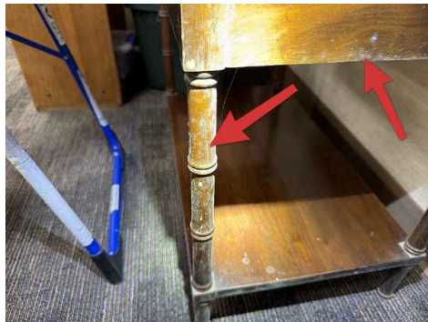
Classroom 3 : suspected mold growth observed
