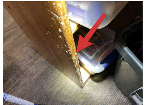
Classroom 3 : suspected mold growth observed
