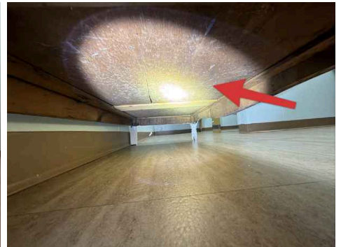
Women's Restroom 1 : suspected mold growth observed
