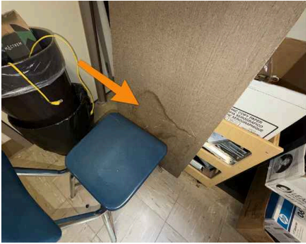
Library Storage : water impacted material observed
