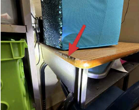
Classroom 2 : suspected mold growth observed
