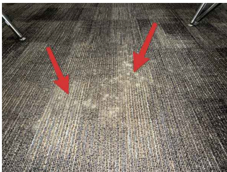
Classroom 2 : suspected mold growth observed
