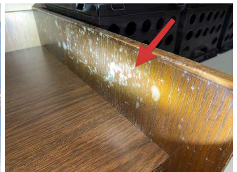
Classroom 7 : suspected mold growth observed
