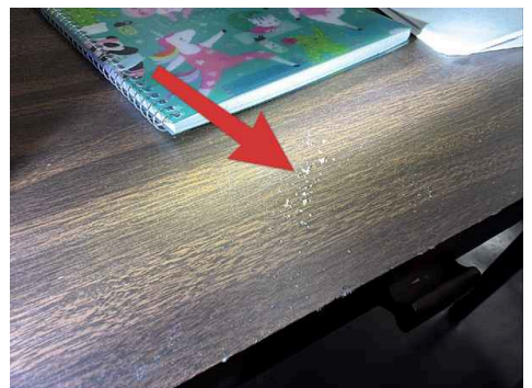
Classroom 6 : suspected mold growth observed
