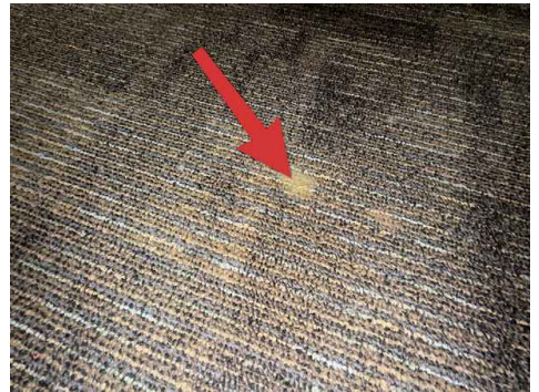
Classroom 2 : suspected mold growth observed
