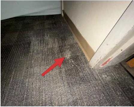
Hallway : suspected mold growth observed
