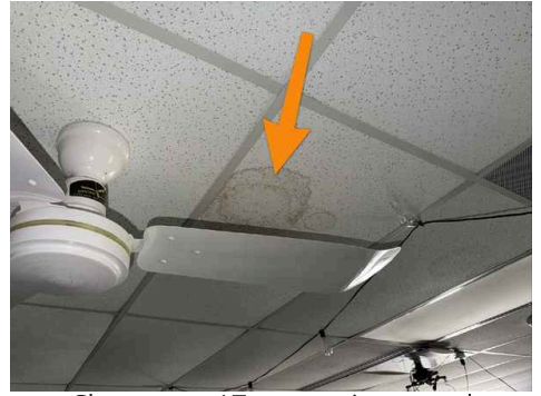
Classroom 17 : water impacted material observed
