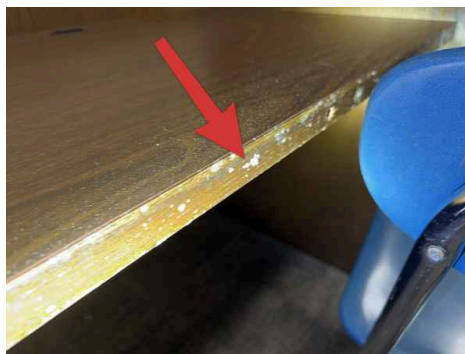
Classroom 7 : suspected mold growth observed
