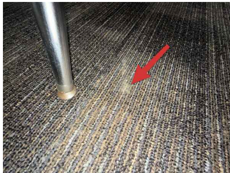
Classroom 14 : suspected mold growth observed
