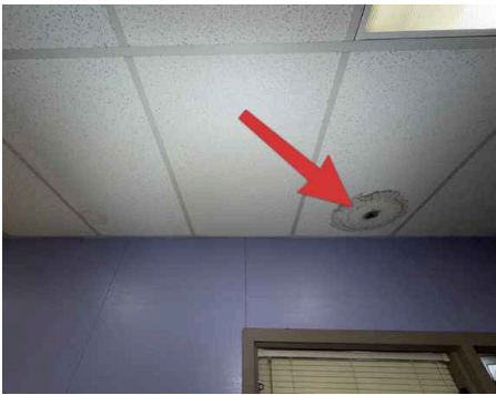
Library Work Room : water impacted material and suspected mold growth observed
