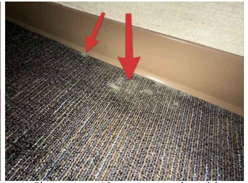
Classroom 13 : suspected mold growth observed
