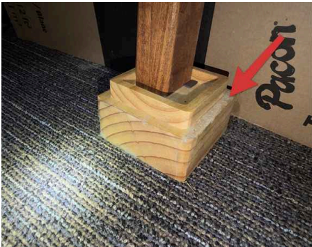
Counselor's Office 2 : suspected mold growth observed
