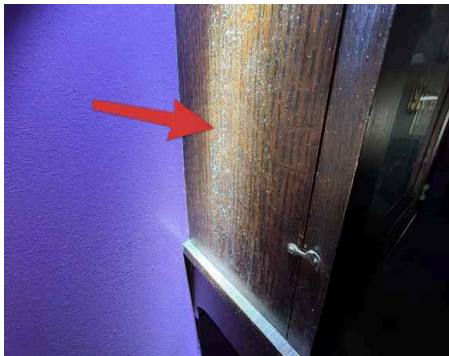
Main Office : suspected mold growth observed
