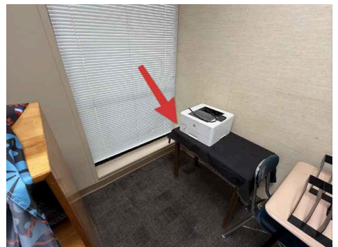
Classroom 1 : water impacted material and suspected mold growth observed
